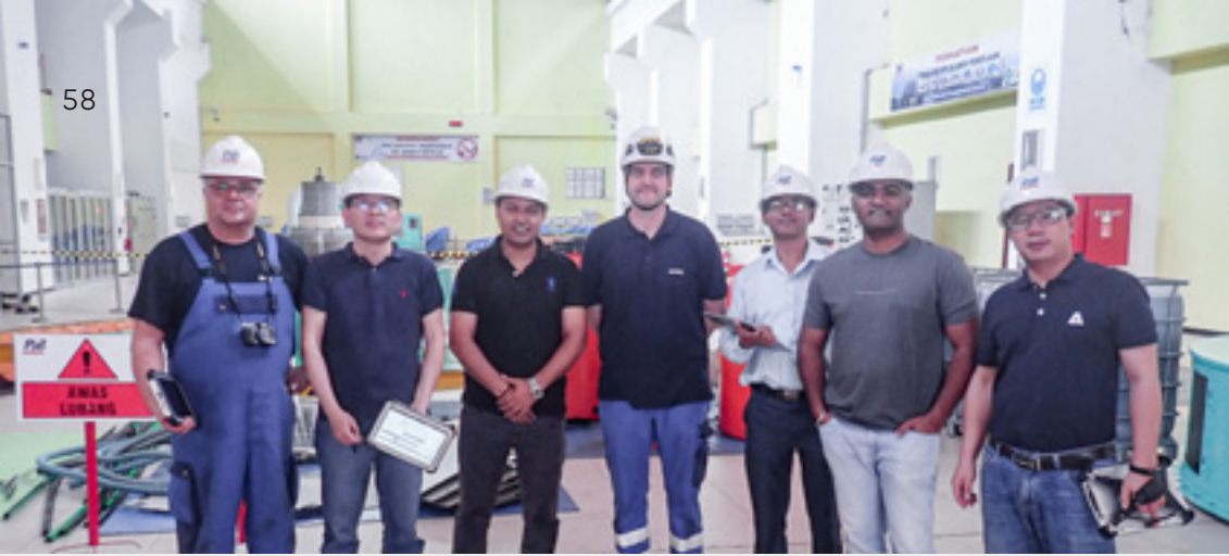
ANDRITZ Hydro experts during on-site inspection using HPP Assessment Tool on dedicated tablets
