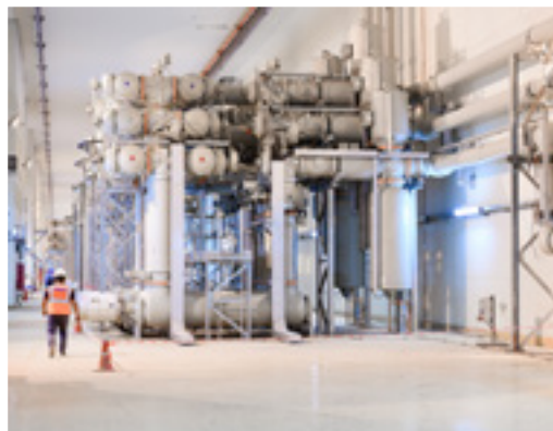
With 1,285 MW, Xayaburi is going to be the most important hydro-electric plant on the Mekong River.
