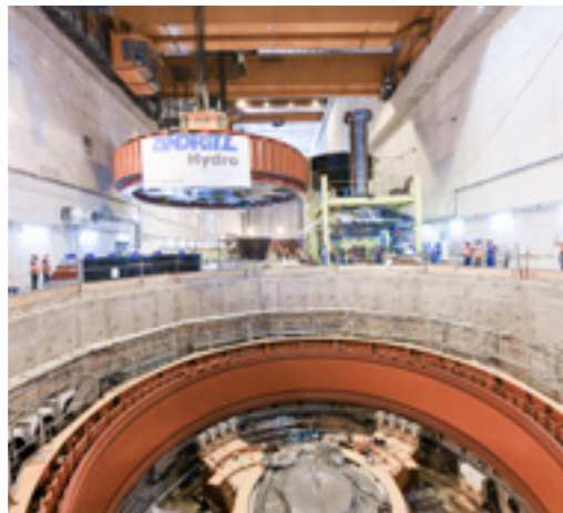
Installation of the generator rotor into the generator pit requires absolute precision and know-how.
